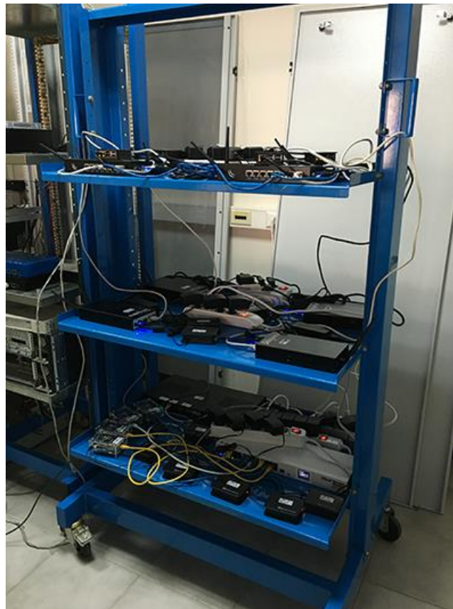
Figure 14. UMOBILE testbed - physical installation
